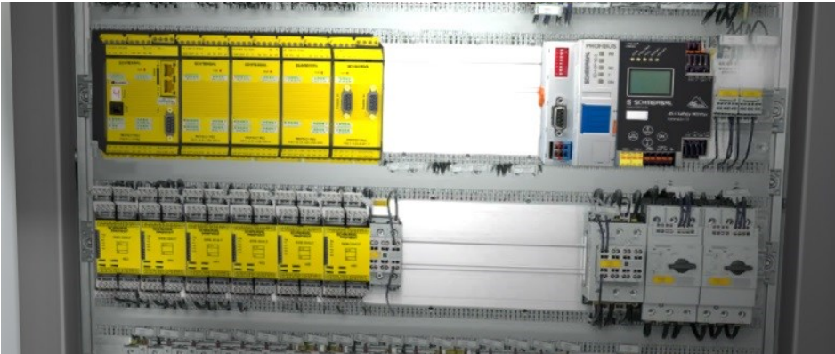
Image 2: Streamlined control cabinet with safety PLC
