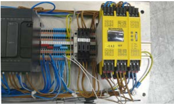
Figure 2: The control unit of the new PUMA bread slicers. On the right of the picture: the PROTECT SELECT OEM compact safety controller.
