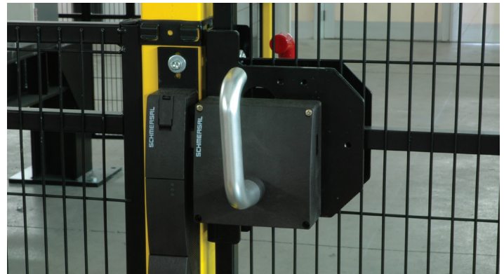
This door lock has an emergency release handle inside the robot cell.
